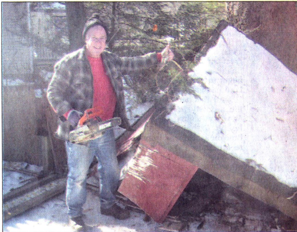
Peter Brady, of the Handy Dandy Handyman Ministry, finishes off the demolition of a garden shed at the home of Denise Gearin in New Milford.
